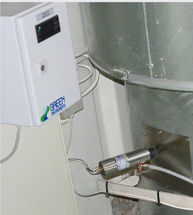
An installation of a G1000 Smoke Density Monitor with the monitoring unit and one optic head
